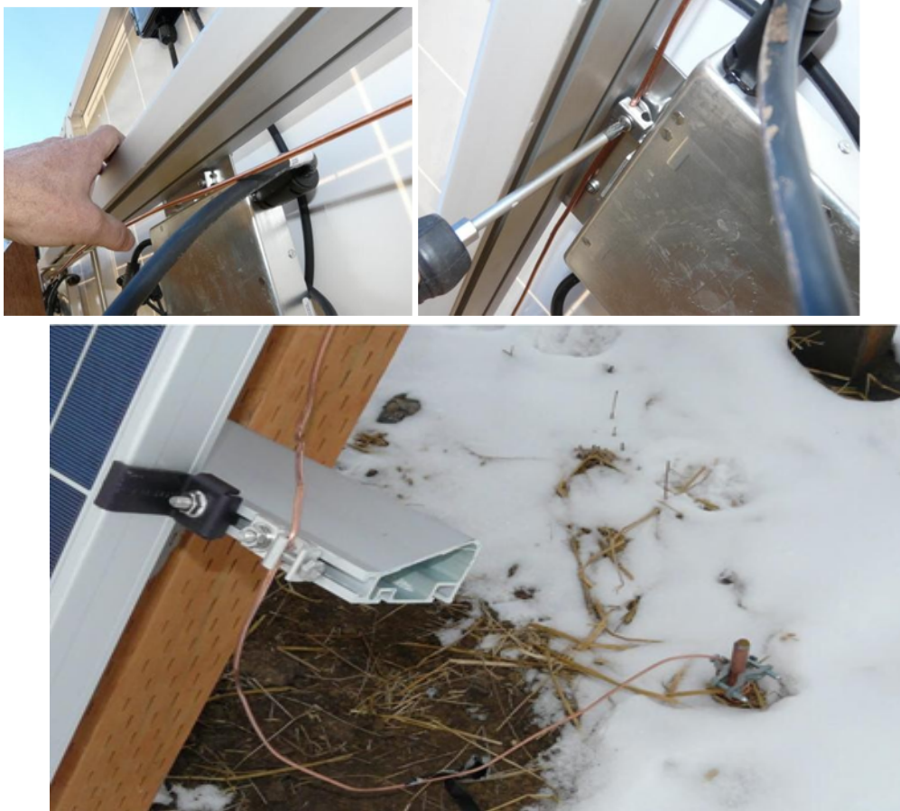
Picture 2.1: Grounding of metal carrier system legs
