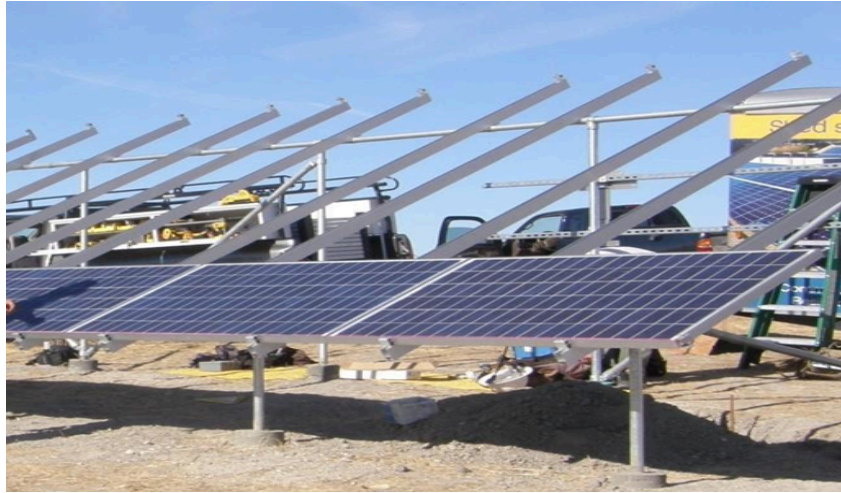
Picture 4.2: Solar panels laid on profiles
