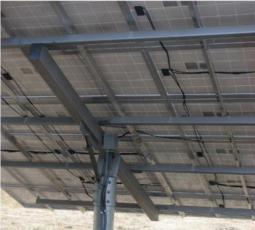
Figure 4.6: Cable transitions between panels
