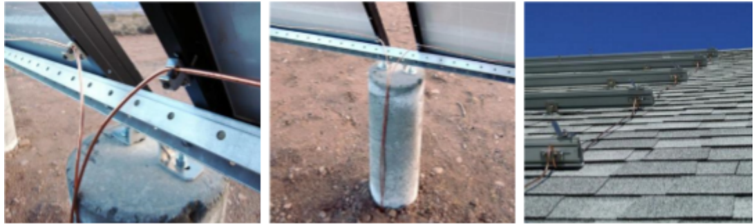
Picture 1.7: Grounding of solar panels in open areas and buildings
