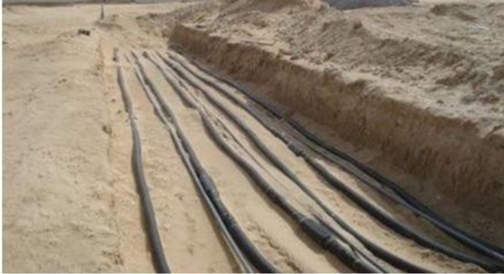
Picture 1.1: Power cables lined up side by side in the channel in the solar power plant
