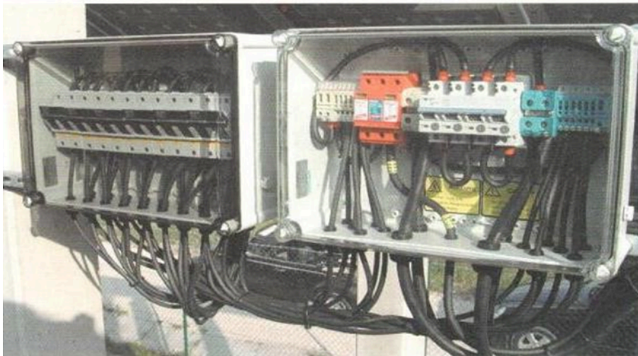
Picture 1.7: Junction box and distribution panel connections
