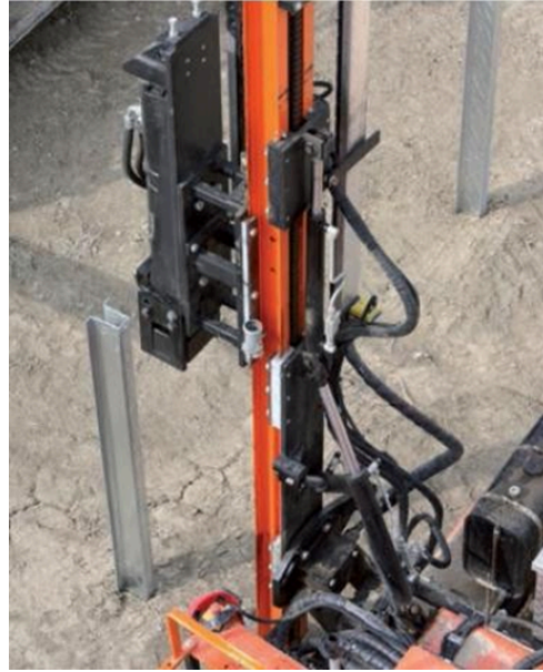
Picture 1.3: Steel foundation piling and driving machine used in solar power plants
