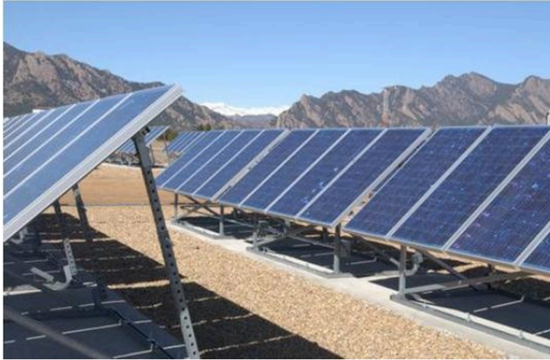
Picture 1.5: Inclined placement of solar panels to receive the sun's rays vertically
