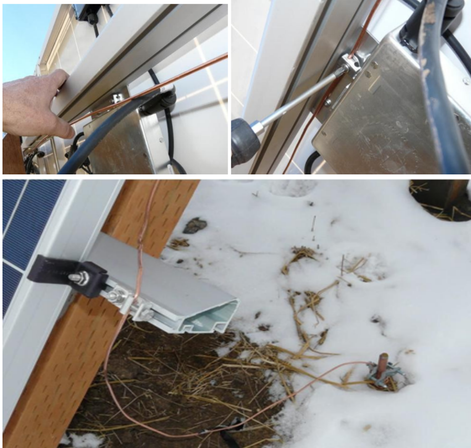
Picture 2.1: Grounding of metal carrier system legs
