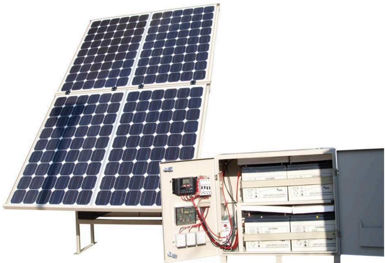
Picture 1.1: Solar panel system power panel
