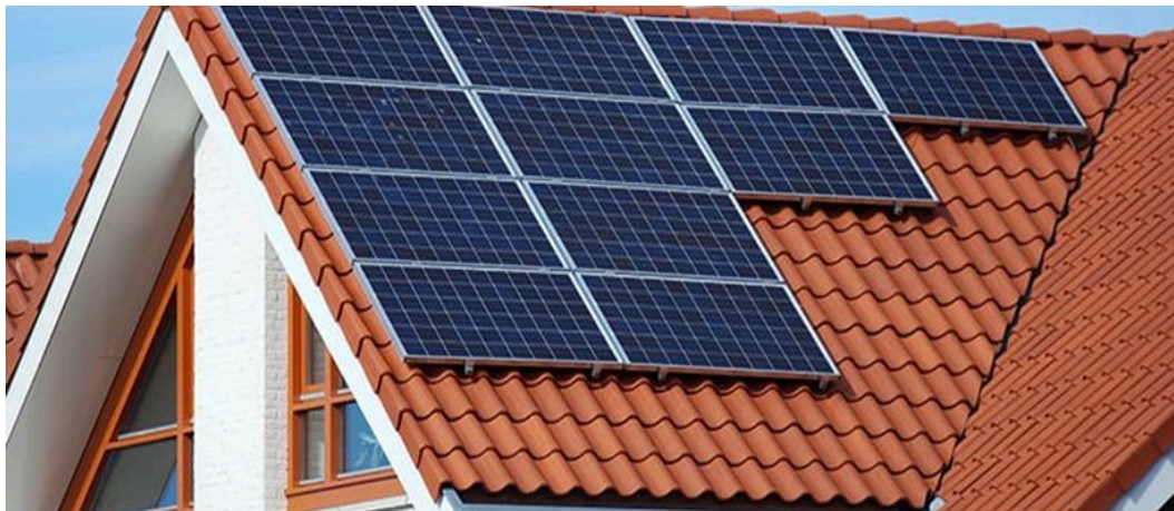
Picture 1.1: Solar panel system facing South
